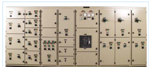
Chiller Control Panel/Main Air Conditioning Switchboard
