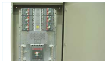
MCCB Pan Assembly Panel Board
