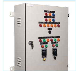
Fuel Pump Control Panel
